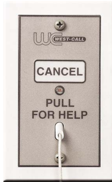
EMERGENCY PULL CORD
