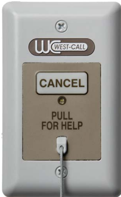
EMERGENCY PULL CORD
